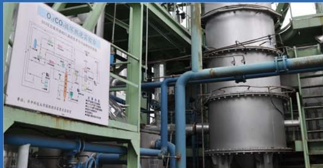
400 kWt Oxy-fuel recycle combustion facility
