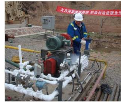
CUCBM CO 2 -ECBM Well Site
