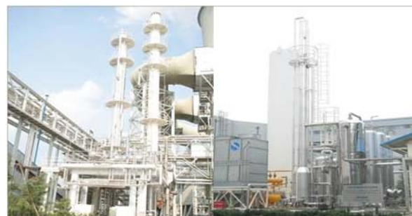
3000 t/a CO 2 capture pilot in Huaneng Beijing Thermal Power Plant
