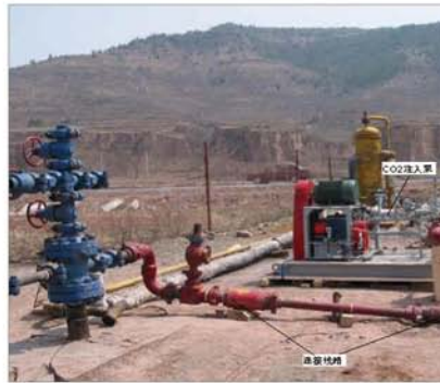
CUCBM CO 2 -ECBM Well Site
