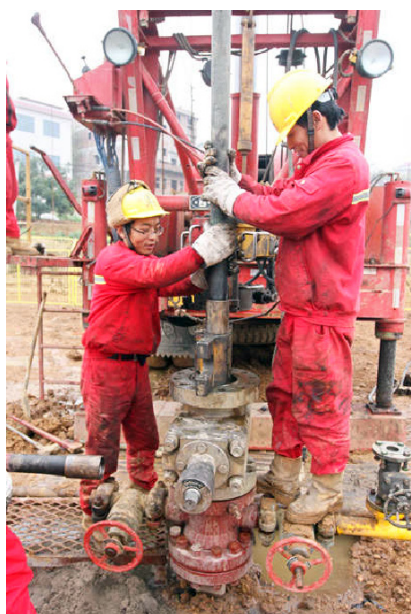
Staff members of Sinopec work on the shale gas exploration well in Qiaotouhe Town, Lianyuan, Hunan Province, on January 7
